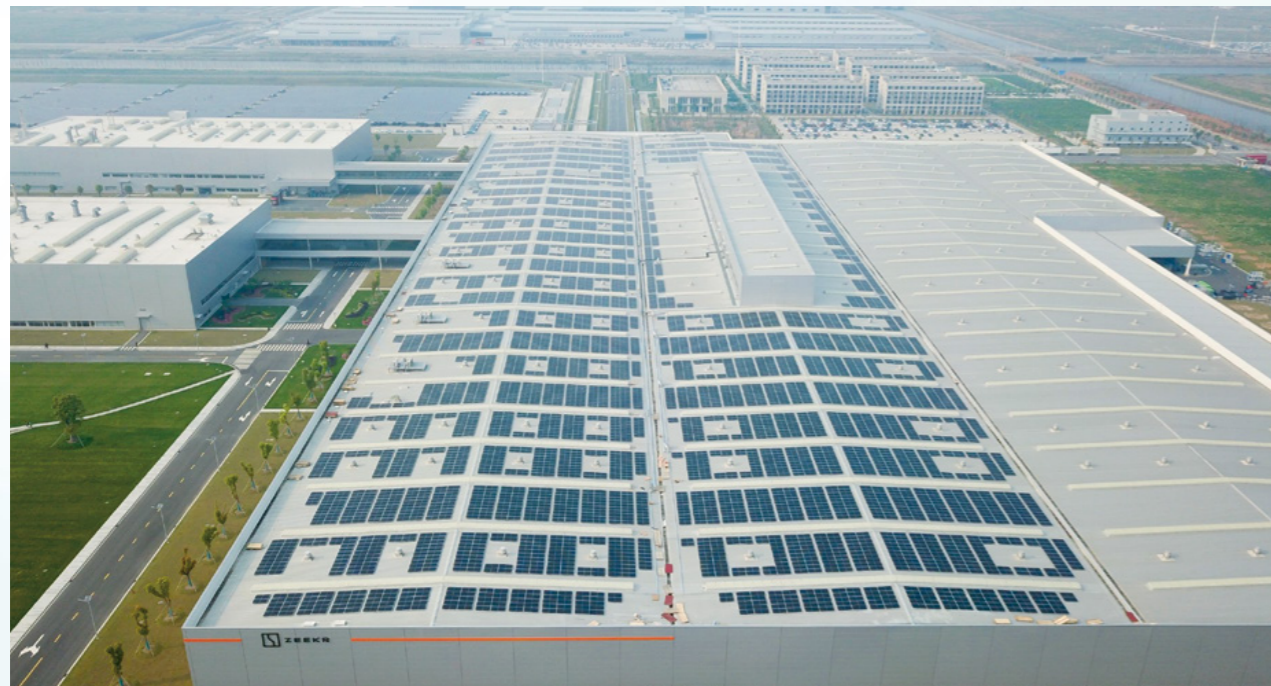
The installed capacity of rooftop photovoltaics in ZEEKR's factory reached 29.46MW. Besides PV systems, ZEEKR's factory will also fully implement green-electricity-certified procurement starting in 2022.
