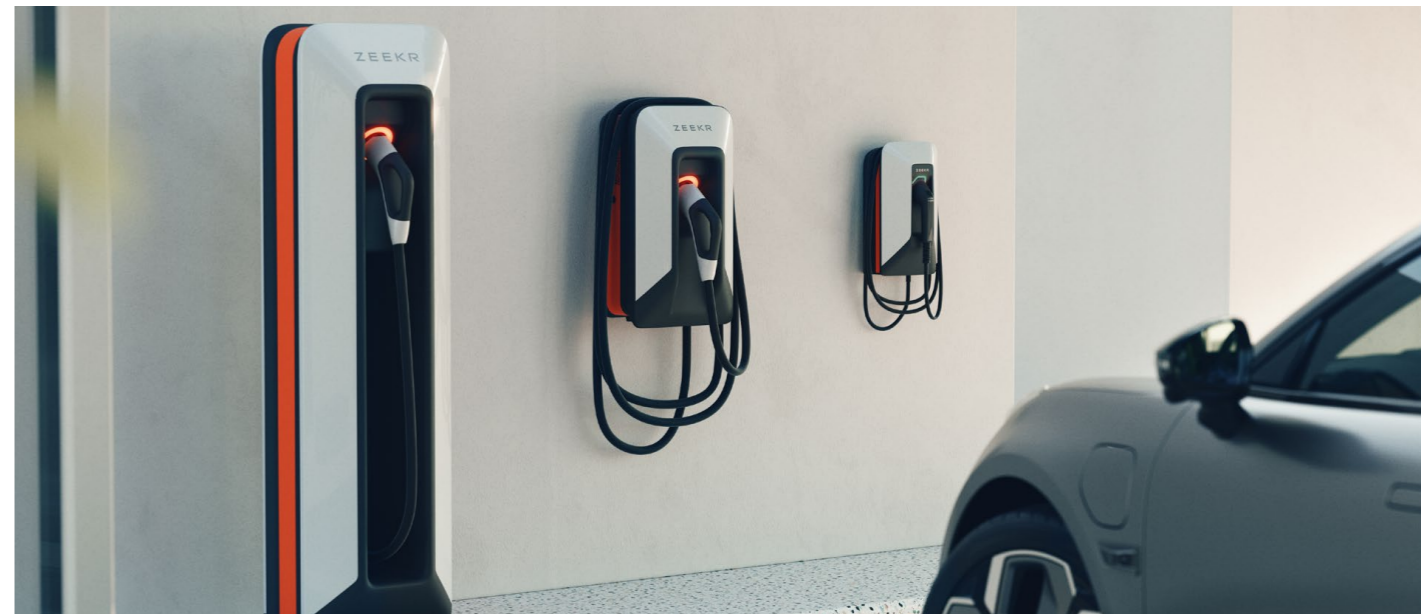
ZEEKR battery charging station
